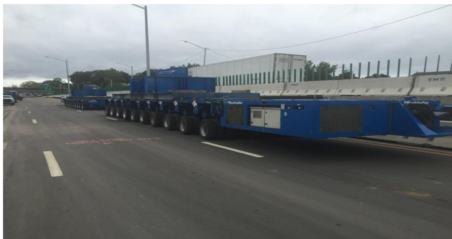
Self Propelled Modular Transporter to be utilized for the remainder of Br. 163 Superstructure Demolition
