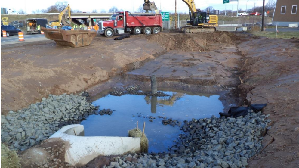
Excavation for new storm water detention basin – East of Ella Grasso Blvd.
